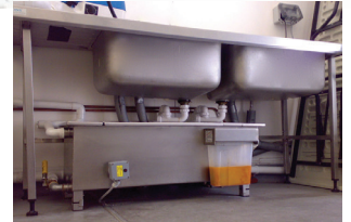
Grease trap and sewage
